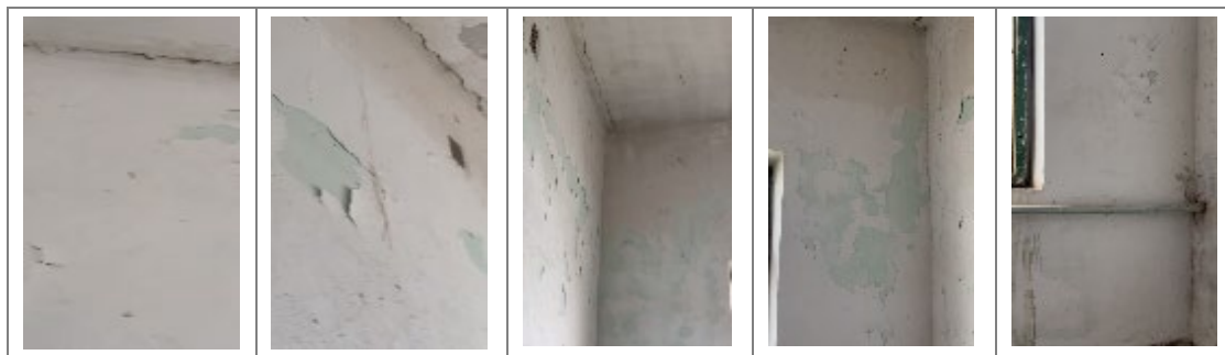
(c) Flooring Condition, Field Mission in December 2024:
