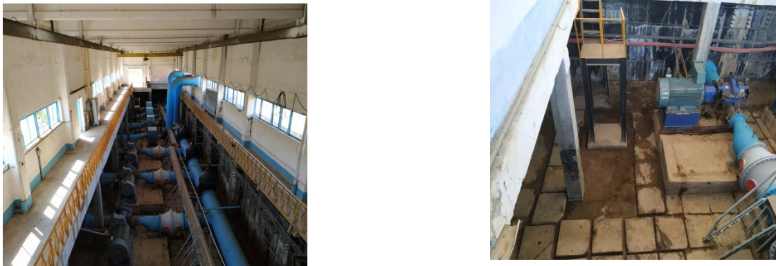
Figure 3.5: Ibn Sino Pumping Station
