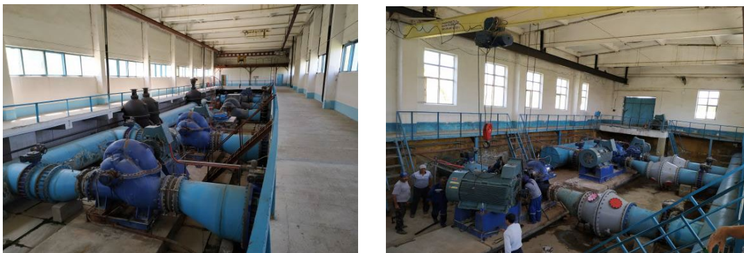
Figure 3.7: Pumping stations of II and III lift
