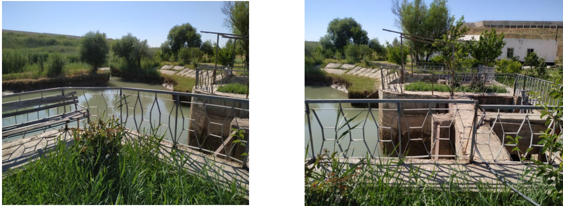
Figure 3.4: Pumping Station Water intake
