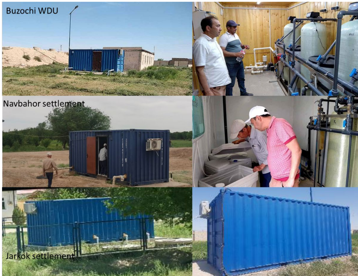
Figure 8: Filtration facilities in Buzochi, Navbahor, and Jarkok (Source: Field visits, May 2023)
